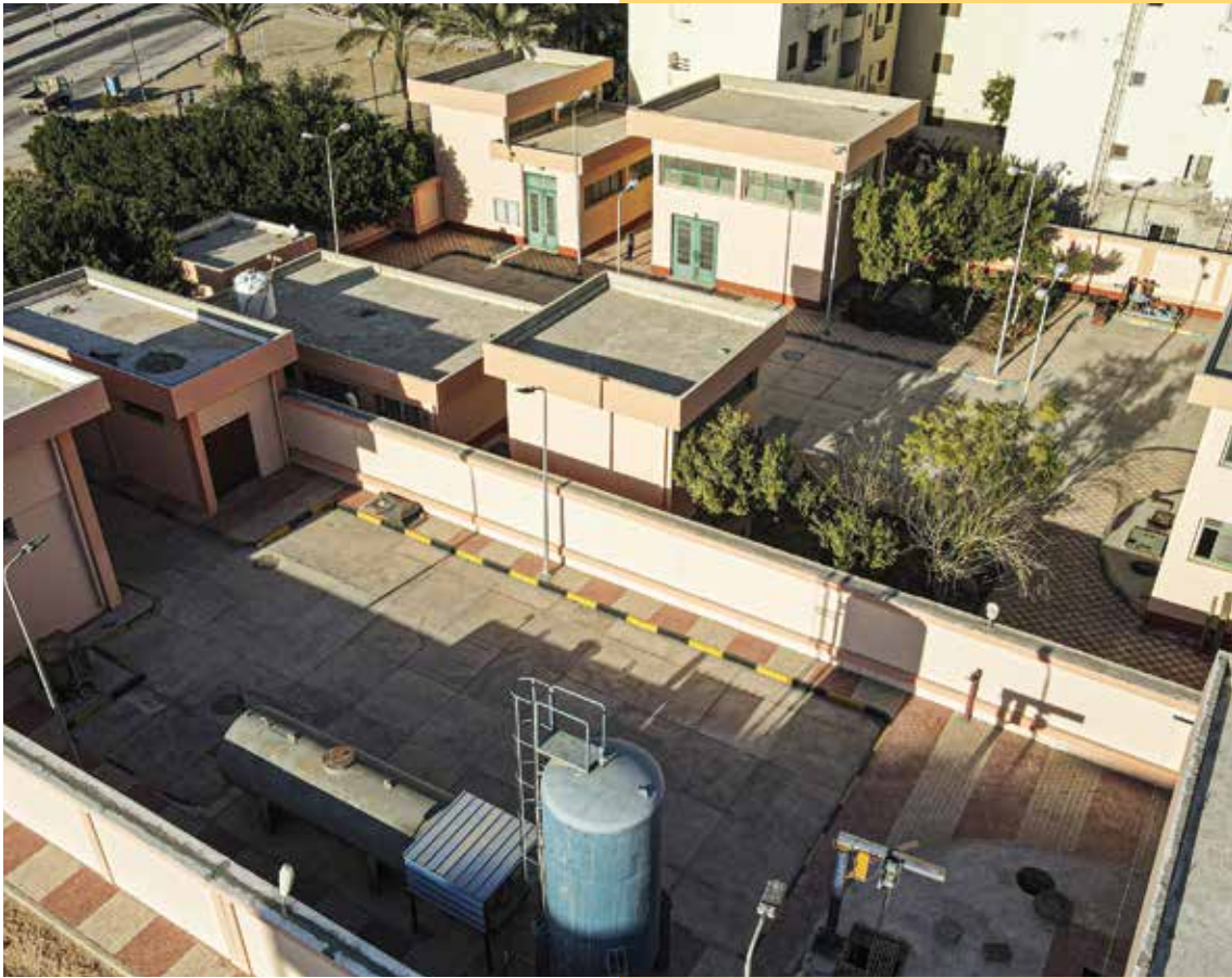
Sewage water pump station-Hurghada National Organization for Potable Water & Sanitary Drainage (NOPWASD)
